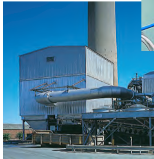
Opacity monitoring on a municipal waste incinerator
