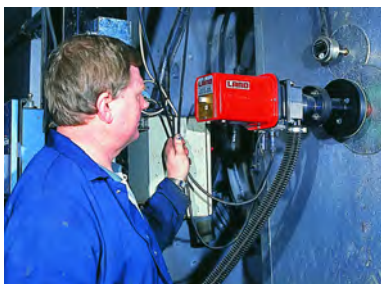
Dust monitoring on a coal-fired boiler
